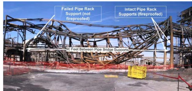
Figure 4 – Collapsed Pipe Rack as a Result of Heat from a Jet Flame.
