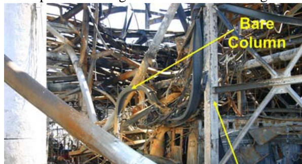
Figure 8 – Collapse of Non-Fire Proofed Structural Steel
