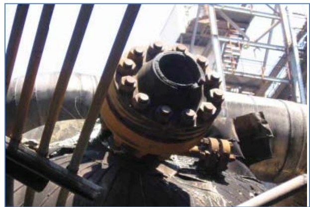
Figure 10 – 8” NPS Hydrogen Piping Severed
